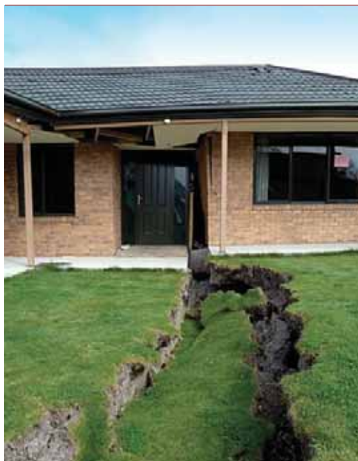
Figure 10: Example of a total loss of a residence in the eastern suburbs due to lateral spreading (left). (Photo: Tonkin & Taylor Ltd).
