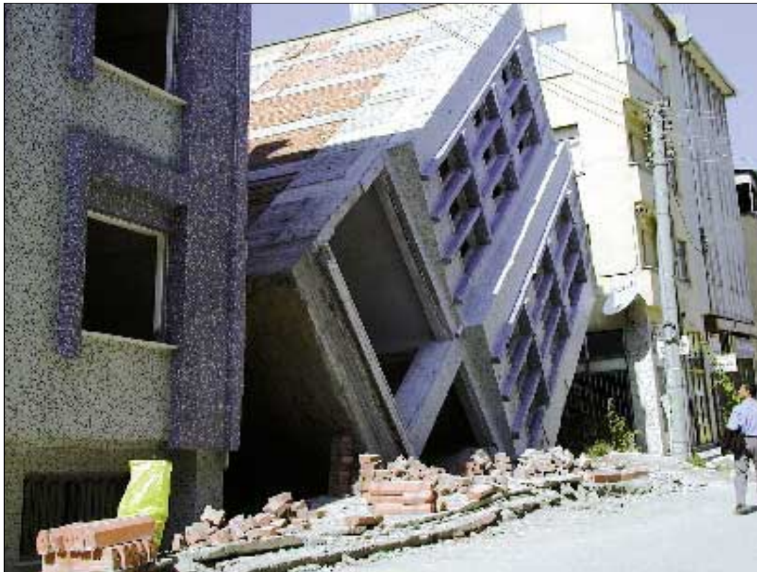
Building overturned due to ground liquefaction and intense acceleration in Adapazari, Turquia.
