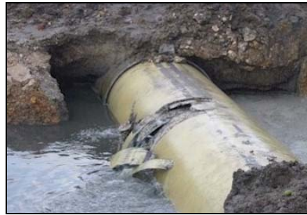
Pipe breakage after trench flooding
