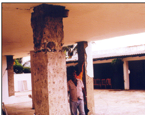
Structural damage. Damaged pillar
