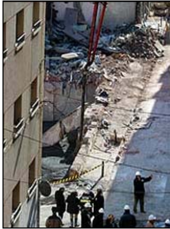
Ground subsidence at El Carmel
