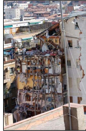
Buildings affected by ground subsidence caused by metro extension works at El Carmel
