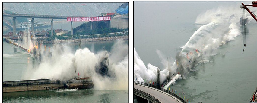
Two moments of a cofferdam demolition (with explosives) at Three Gorges Dam (China)
